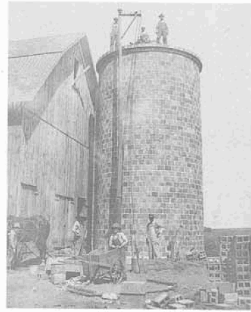
The Building of a Silo—In 1911, putting up a silo was not an easy task. The blocks and mortar were drawn to the top of the silo with a hoist, pulling it up with a horse. Standing on top of the silo by the hoist is George Bayer at the age of 16. His brother, Walter, is by the horse; another brother, Leonard, is by the wheelbarrow. The silo was built on the late Rudolph Bayer farm two miles north and 2½ miles east of Elma. The farm is now owned by Mr. and Mrs. Richard Larsen.
